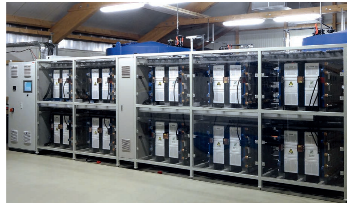
Vanadium Redox Flow Storage Systems.
