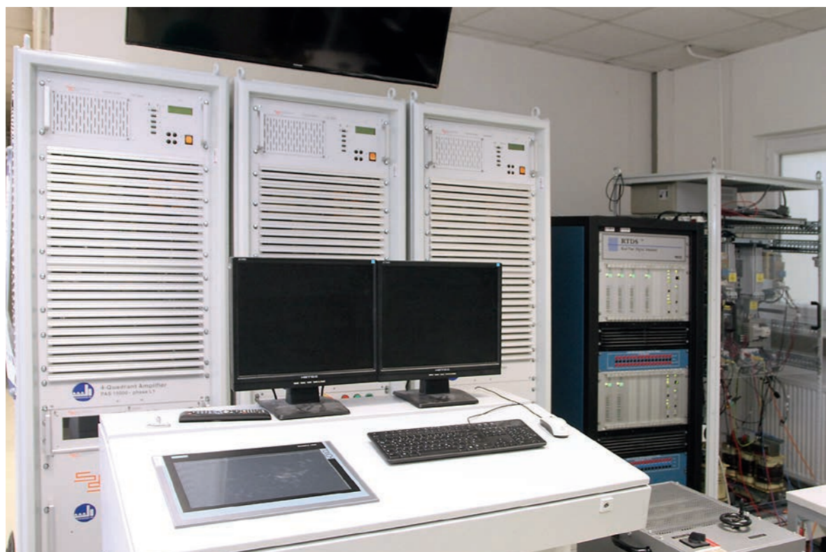
Power-Hardware-In-Loop Setup for Smart Transformer grid test integration.
